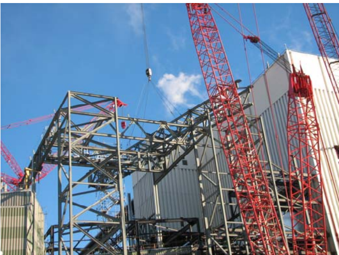
Manitowoc 18,000 crane completes 70 Ton pick for SCR unit while the other 18,000 crane works in the background on the AQCS.
